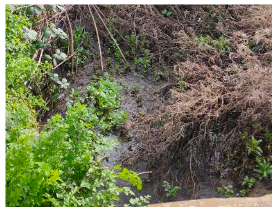
Overgrown Culvert - Start
