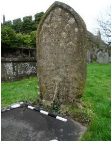
383 – this is the monument which has been braced with timber.
