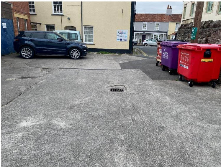
Photo 4 – Shallow rainwater gully to carpark
